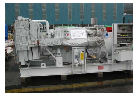
MAN – Dead Ship Generator
